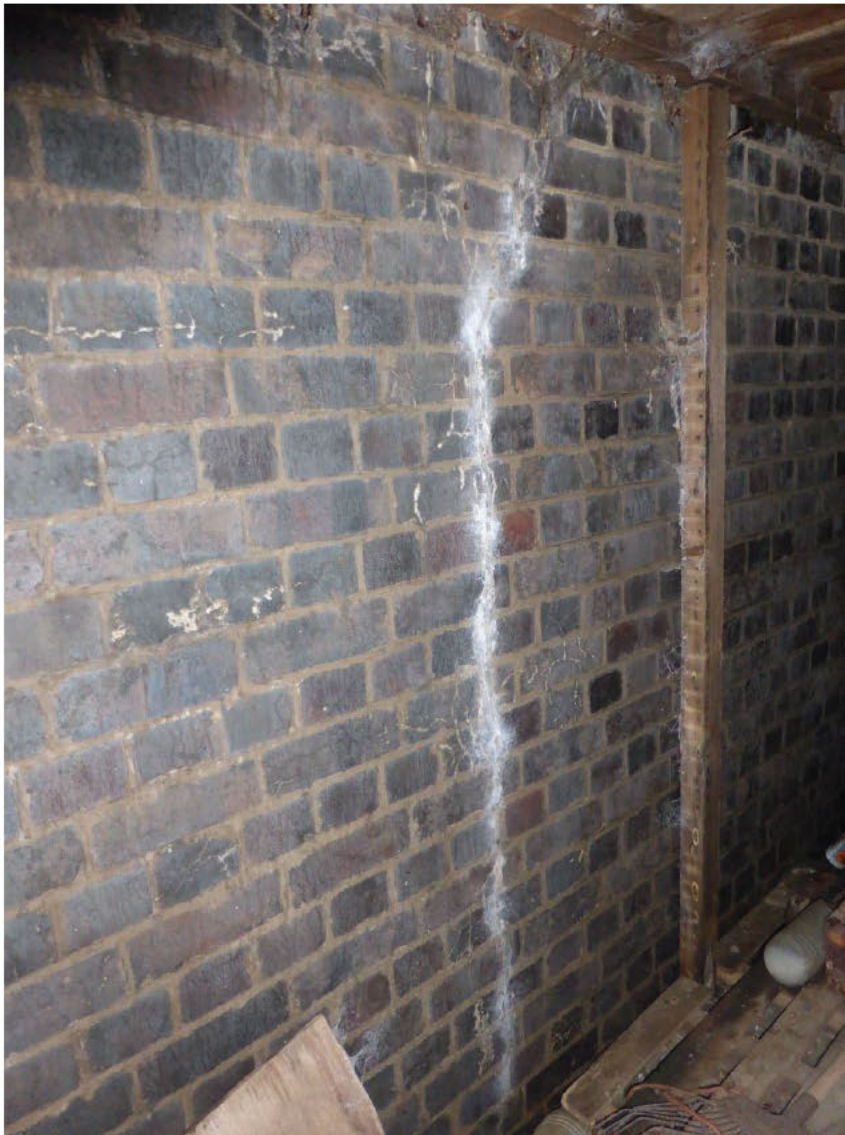
10) North abutment – fracture view behind the shed
