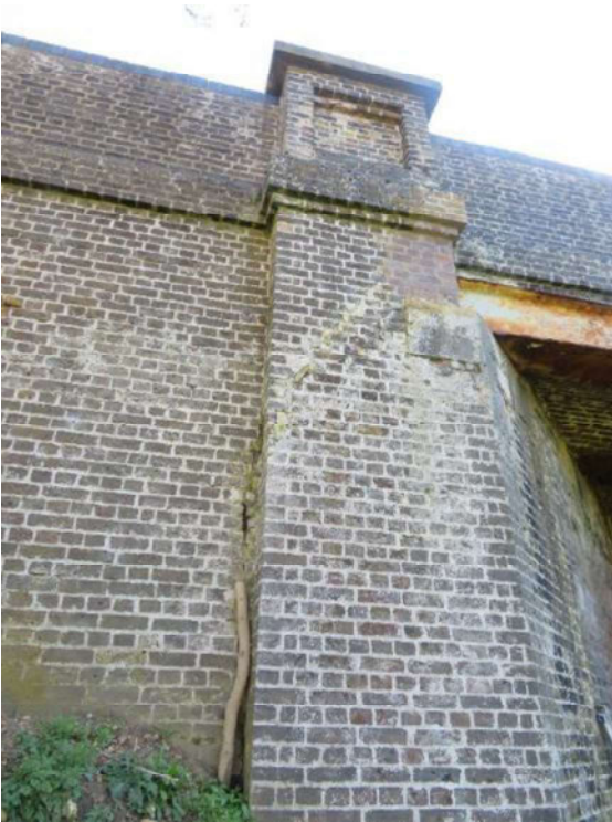
Photograph 33. Northeast wingwall – Vertical fracture
