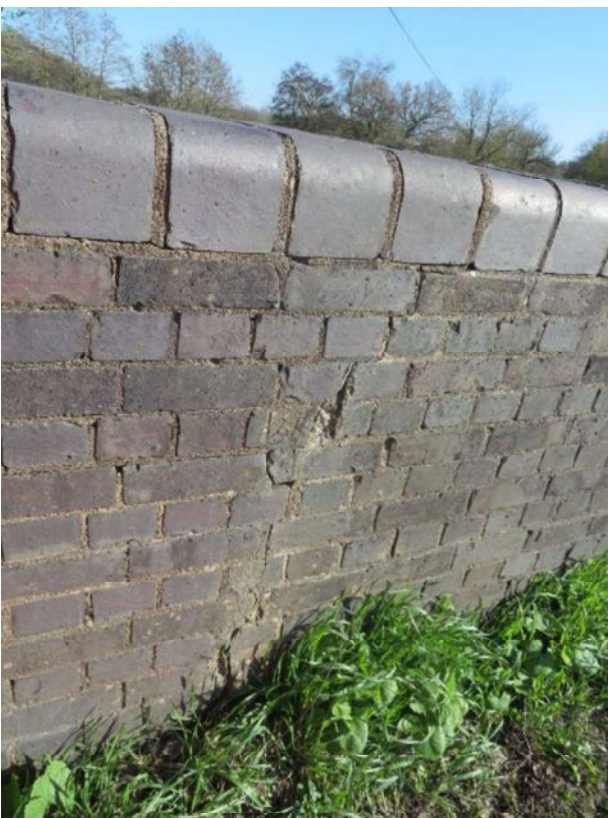
Photograph 40. South Parapet – broken mortar tab
