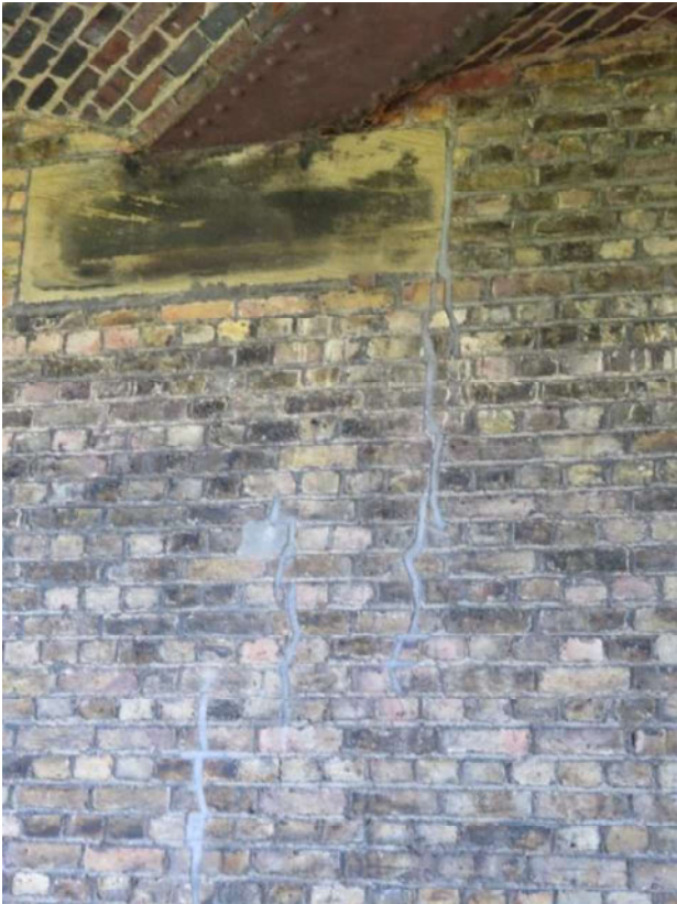
Photograph 28. West abutment – Fracture below second internal girder from south
