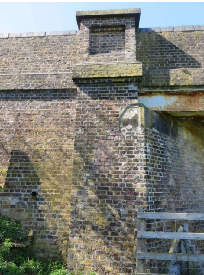
Photograph 34. Southwest wingwall – Fracture
