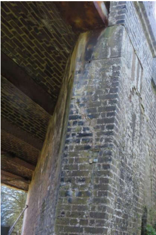
Photograph 29. West abutment – north edge fracture
