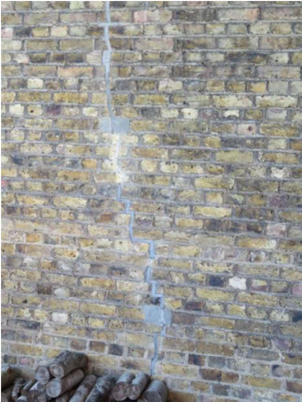
Photograph 27. West abutment – Fracture below second internal girder from south
