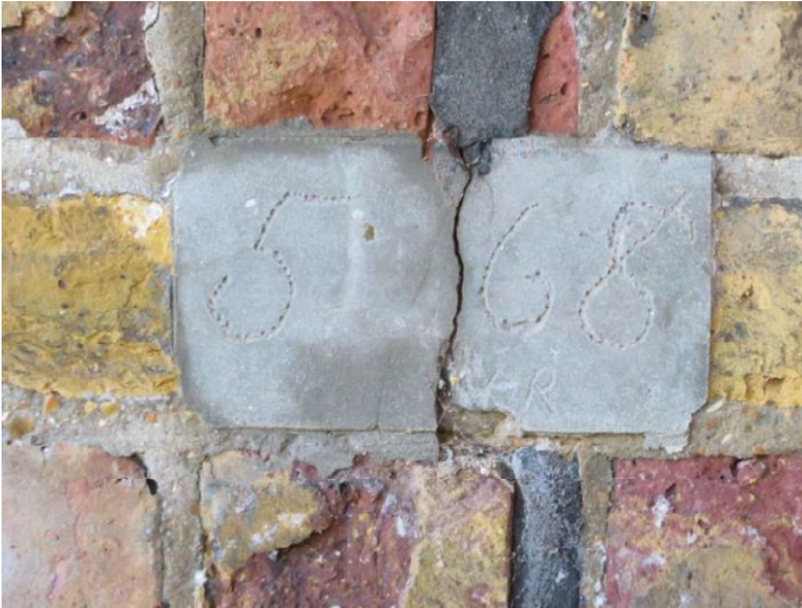
Photograph 31. East Abutment – Vertical fracture under second internal girder from north -broken mortar tab
