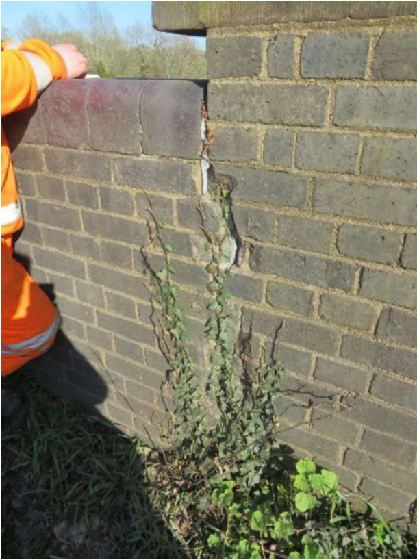
Photograph 41. Southwest Parapet – Filled fracture
