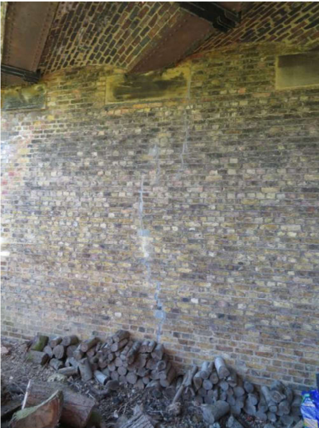
Photograph 26. West abutment – Fracture below second internal girder from south
