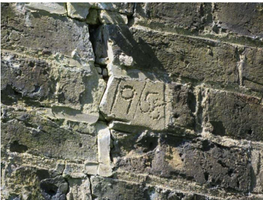
Photograph 36. Southeast wingwall – fracture mortar tab
