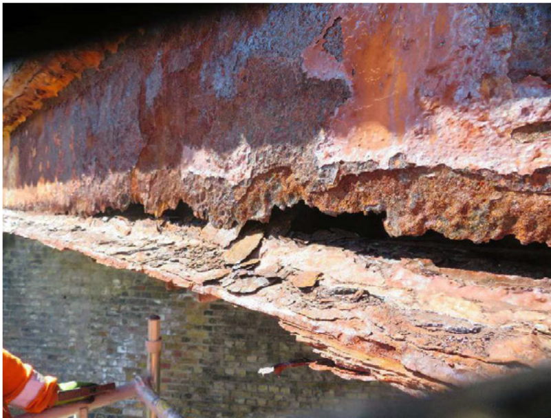
Southeast edge girder at midspan showing severe corrosion
