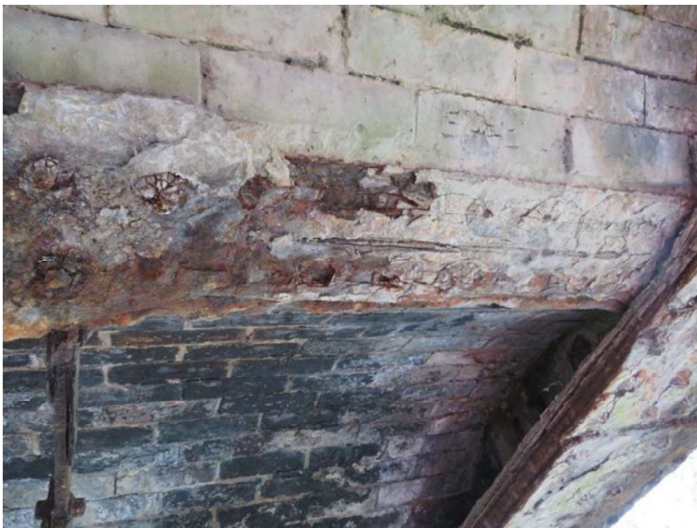
15. Condition of IG3 also showing curtailment of flange plate severely corroded
