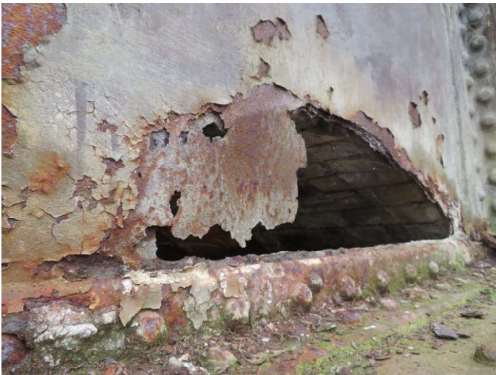
20. Example of sever corrosion on edge girders
