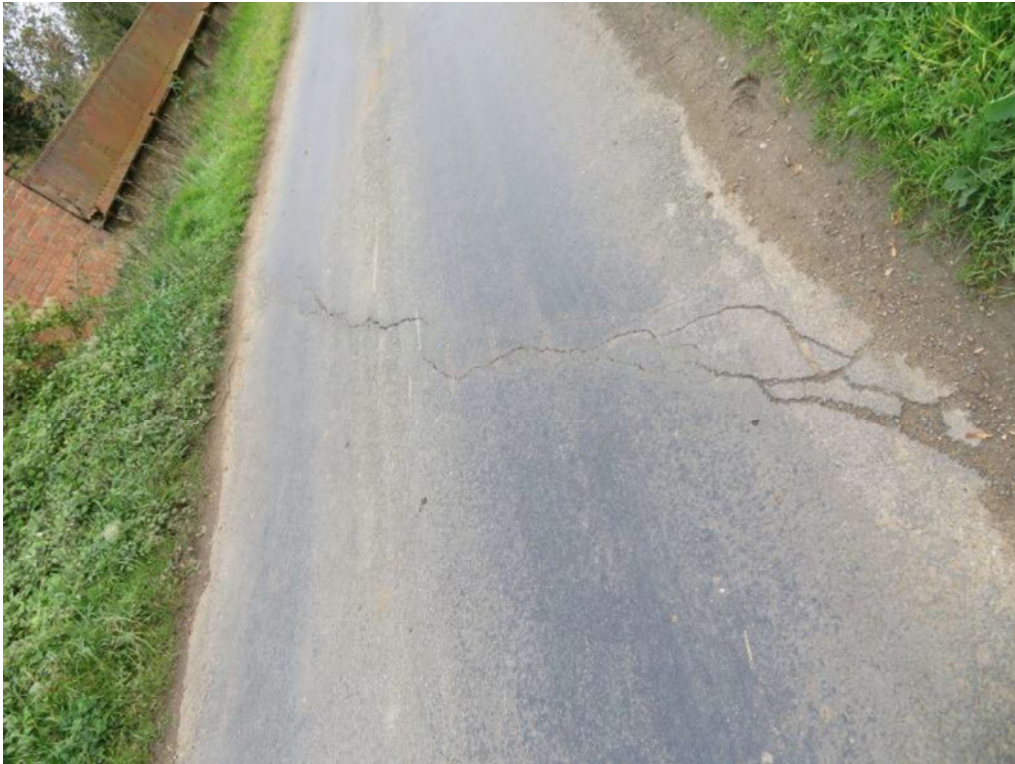
25. Crack and settlement in road surface at west end
