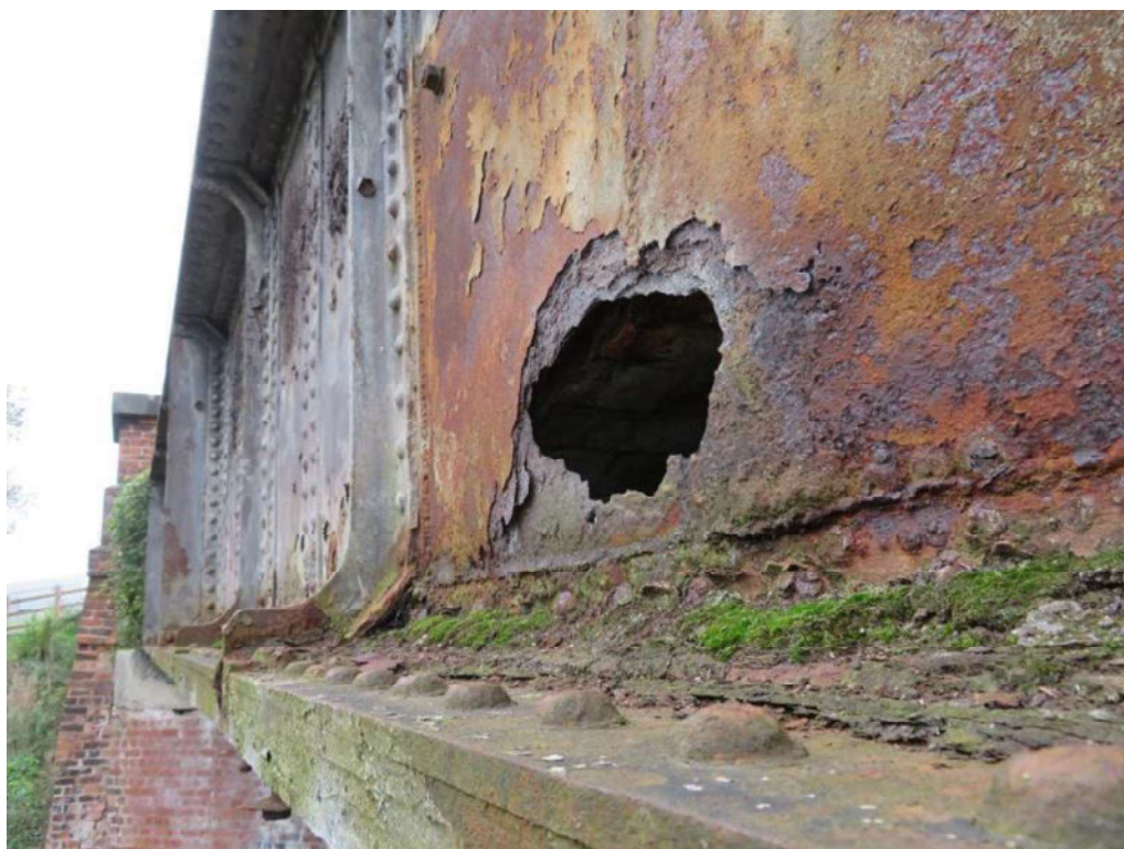
21. Previous repair which has since corroded though
