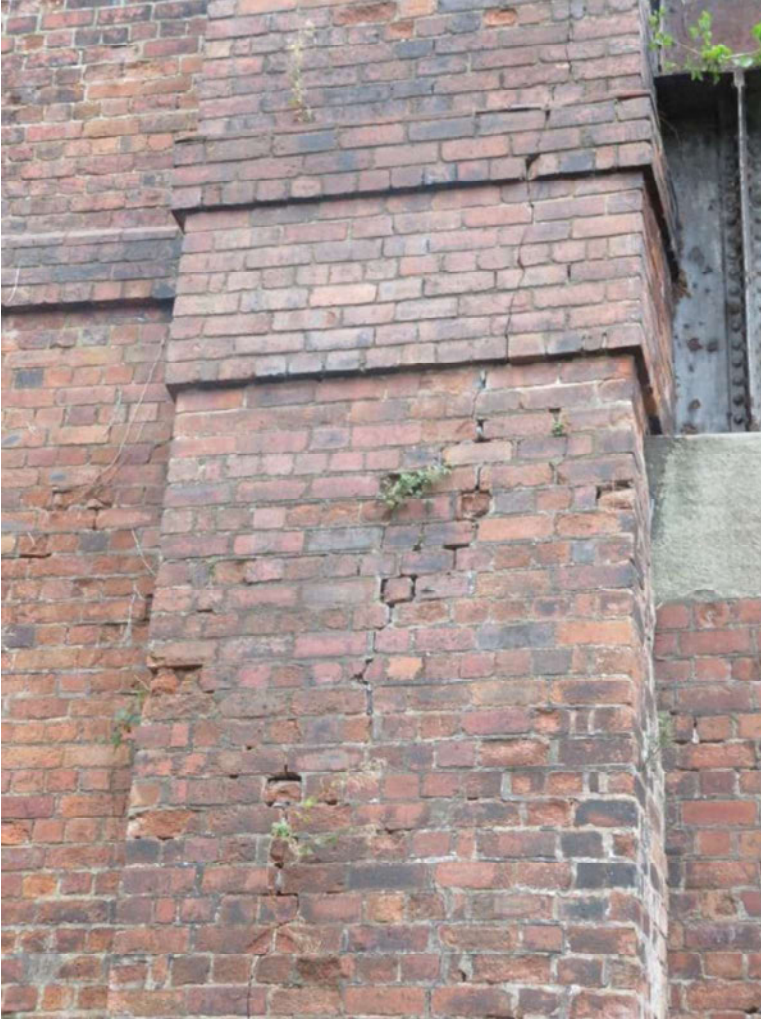
24. Hairline fracture in north east buttress
