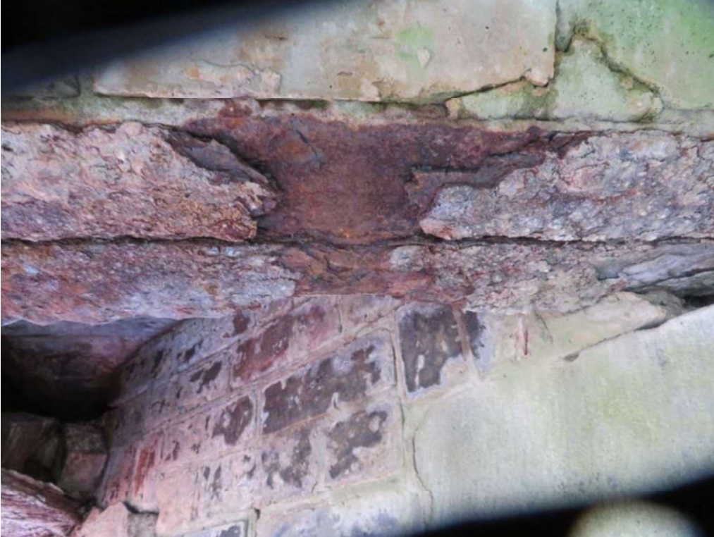
13. Condition of IG1 showing missing angle legs and stained jack arch mortar
