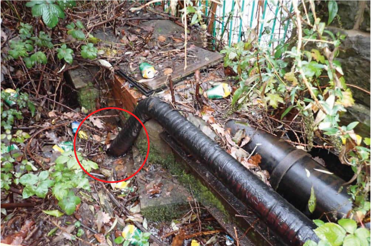
Photograph 25: Water leaking behind south parapet
