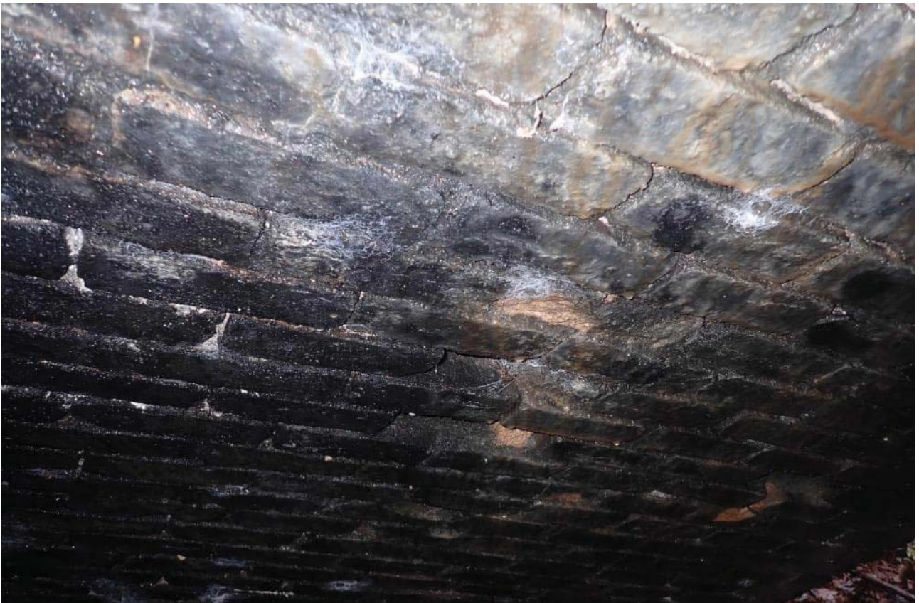
Photograph 22: Mortar loss and spalling to arch soffit
