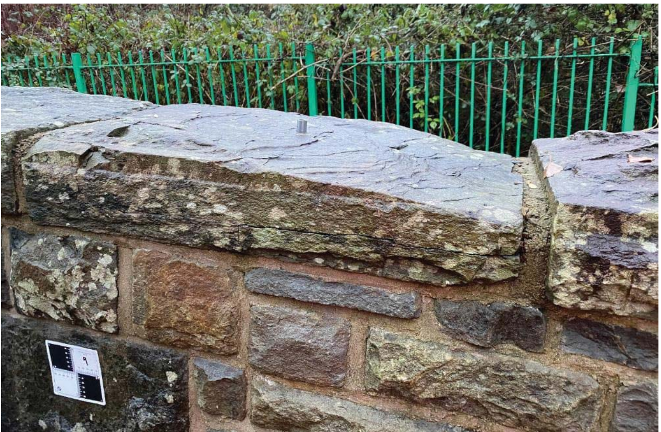
Photograph 28: Steel dowels through cope
