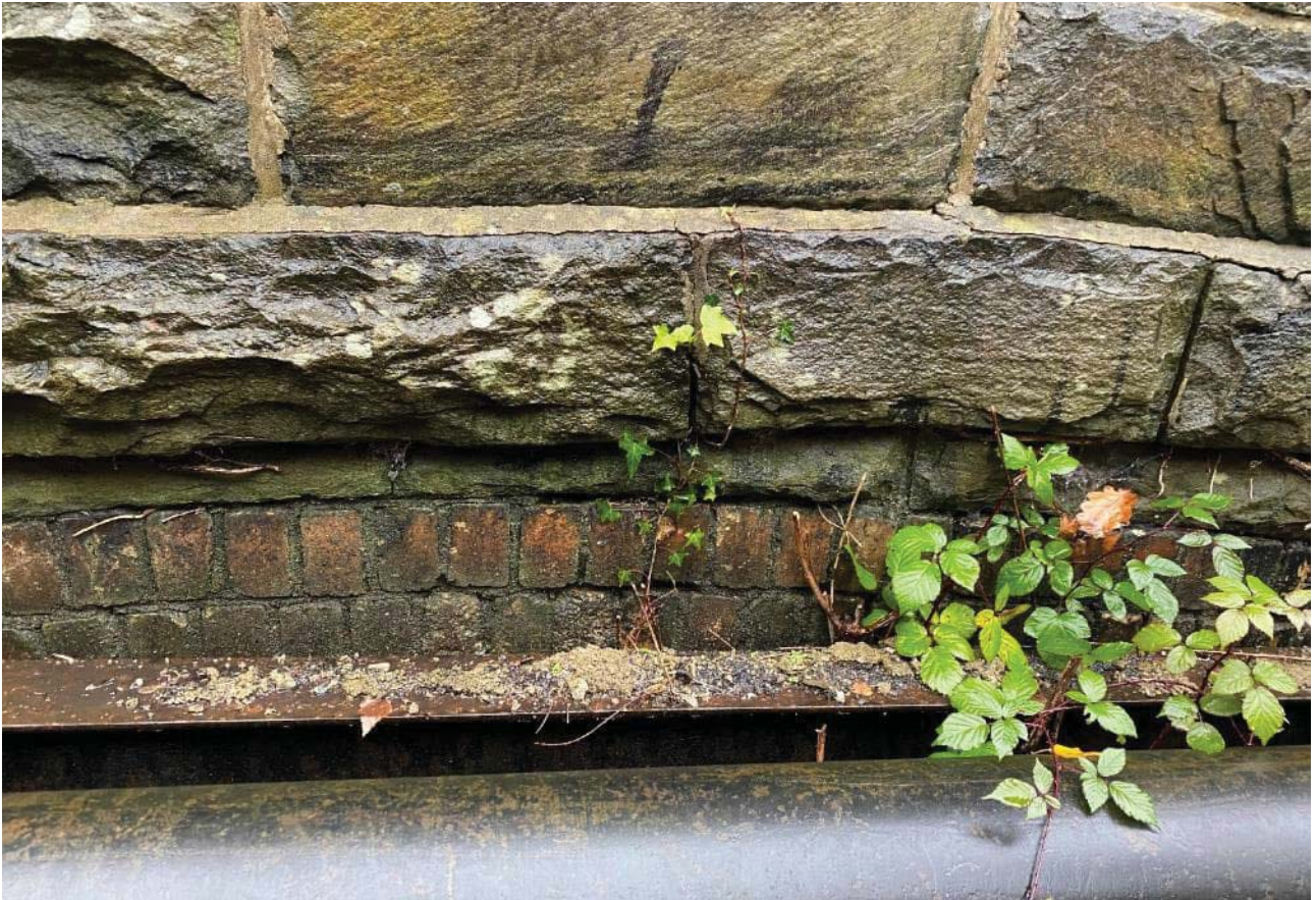
Photograph 24: South elevation arch ring – open joints
