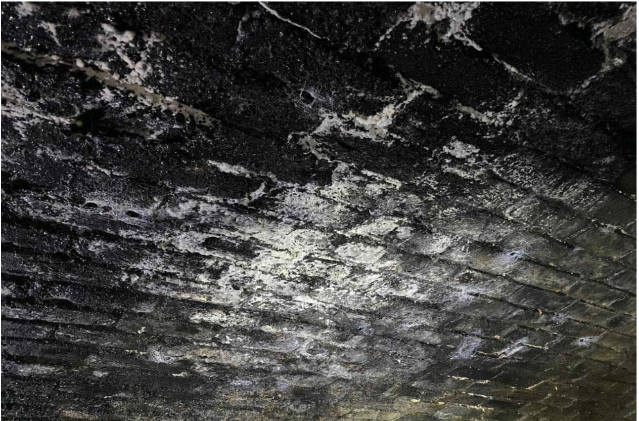
Photograph 19: Arch soffit at crown displaying washout and calcite staining
