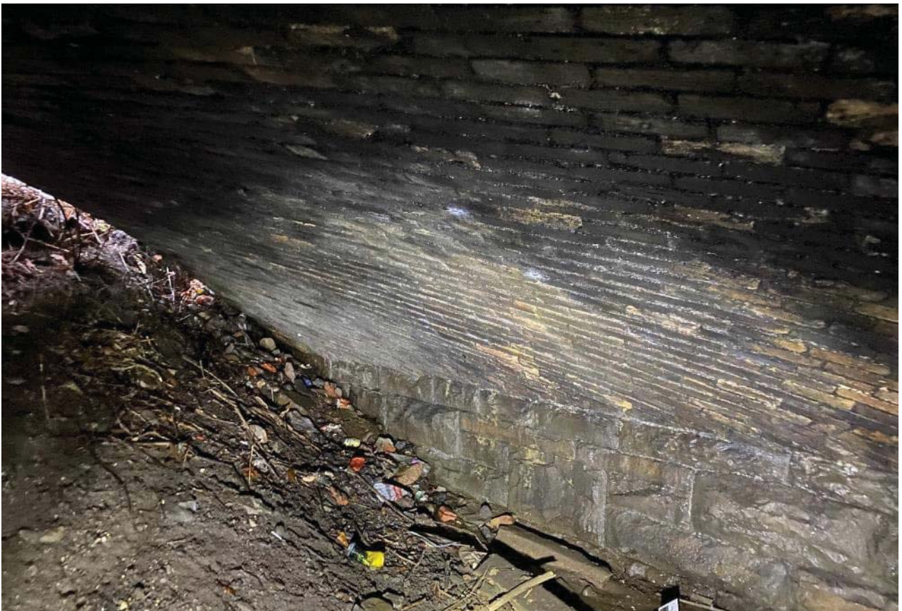
Photograph 6: Soffit at east haunch
