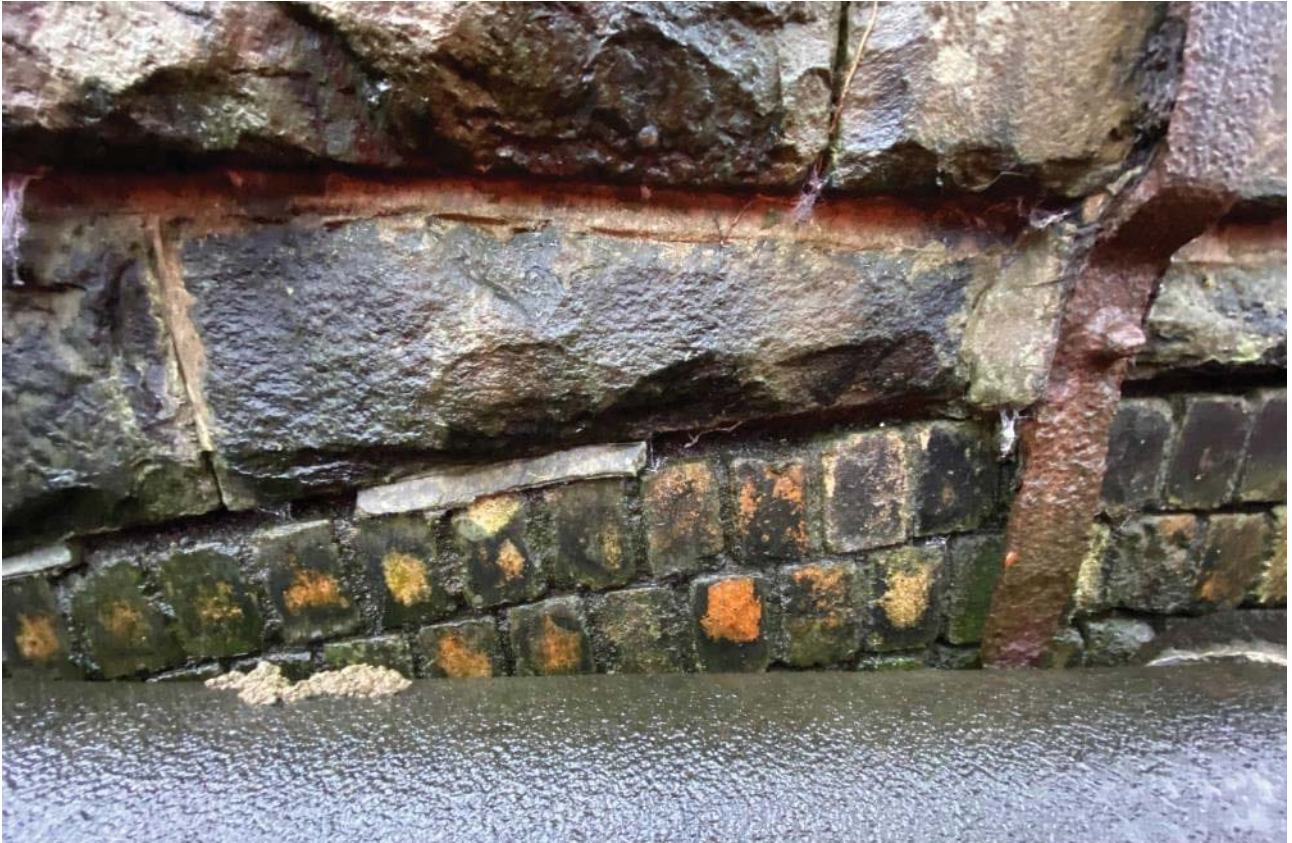
Photograph 23: North elevation arch – open joints
