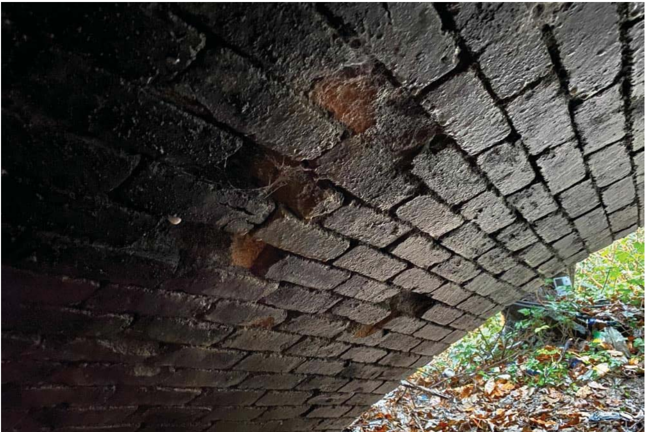
Photograph 20: Spalling to individual bricks north west haunch
