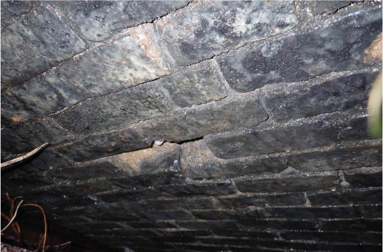
Photograph 21: Individual missing brick to soffit
